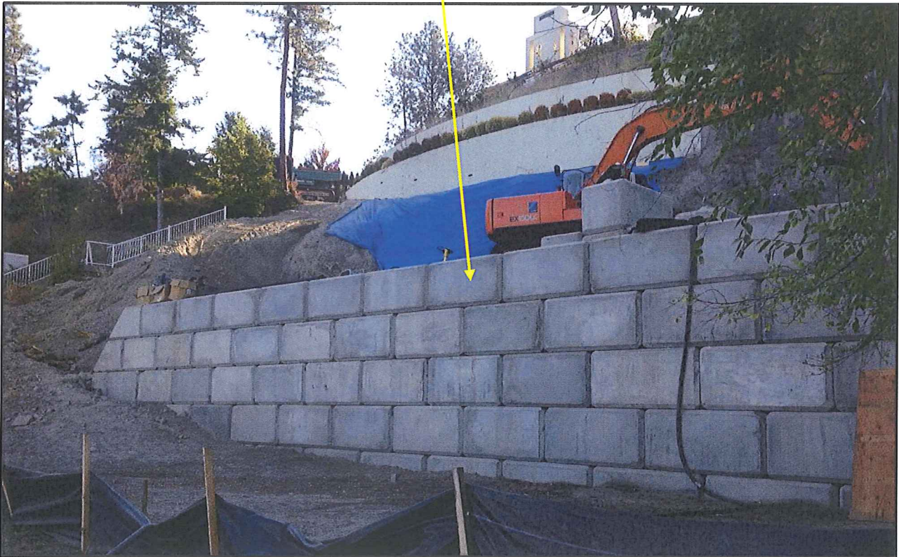
Photo 1: Existing Over-height Lock Block Retaining Walls (from Okanagan Lake High Water Mark)
